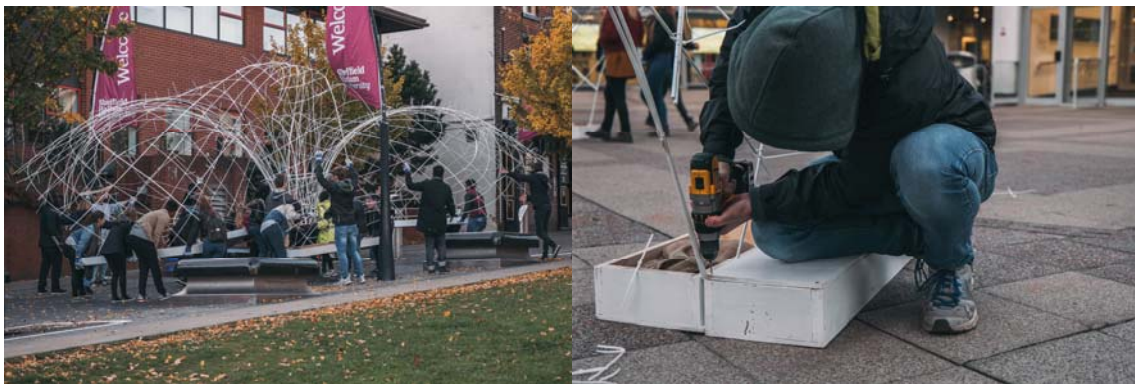
Figure 8 Relocation possible due to low weight. Screwing of bases. (© Matt Bell for SHU)
