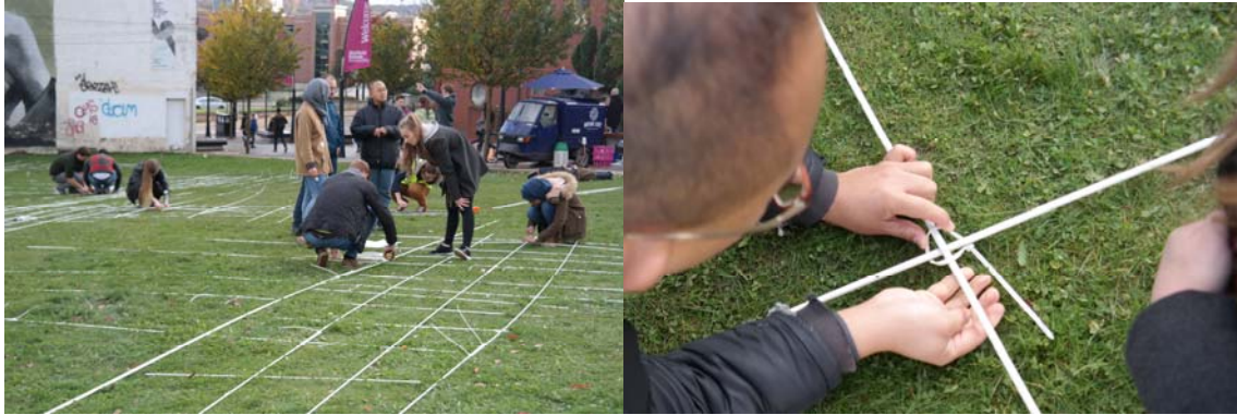
Figure 7 Flat mat assembly at flat grass area and cable ties at intersections (© Edyta Augustynowicz)
